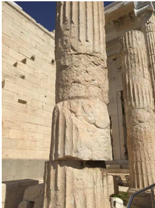
Figure 12. Shear failure between blocks in a multi-drum column located in Acropolis in Athens, Greece.
