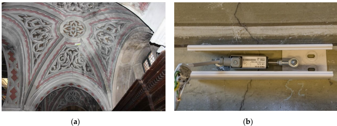
Figure 13. St. Bassiano: (a) monitoring of cracks in a masonry vault by means of (b) LVDT displacement transducers.
