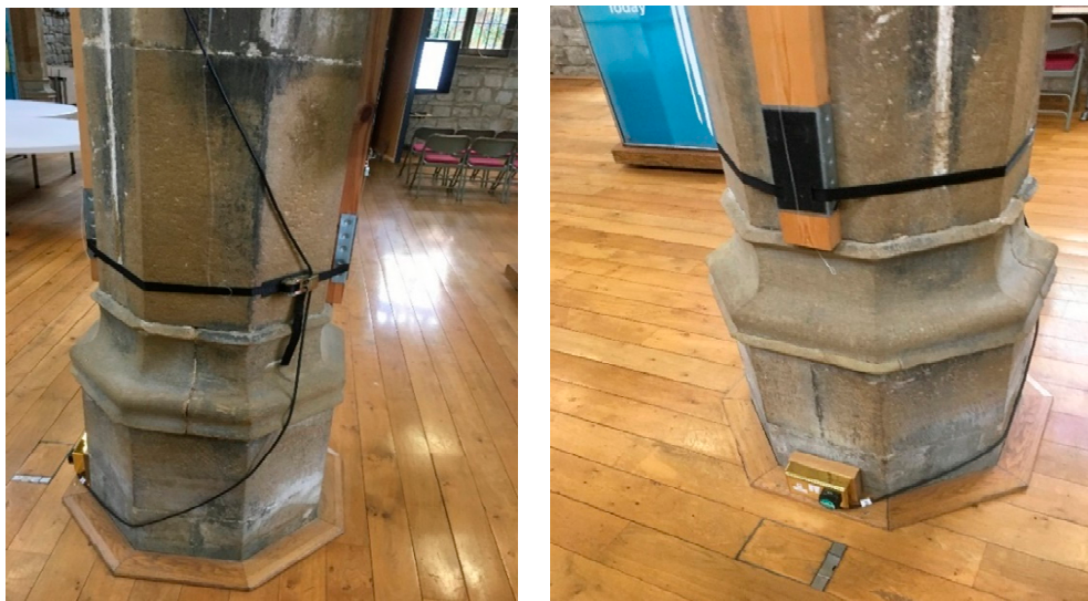
Figure 9. Further changes to Building 2 to provide more usable electric sockets.
