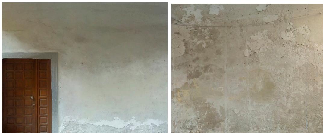
Figure 13. Some orthophotos for the vertical wall (left) and the vault (right). It is now possible to measure areas and to compute the costs of the interventions.
