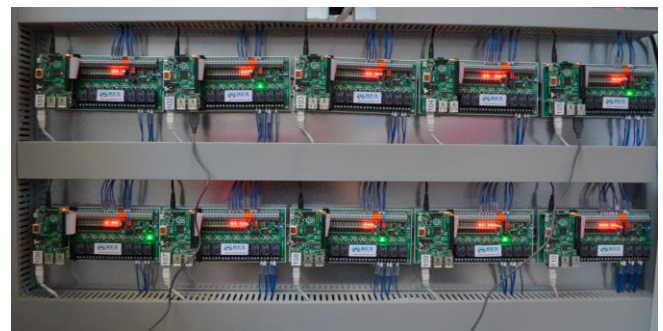
Fig. 4. RTUs installed on INCAS pilot line
