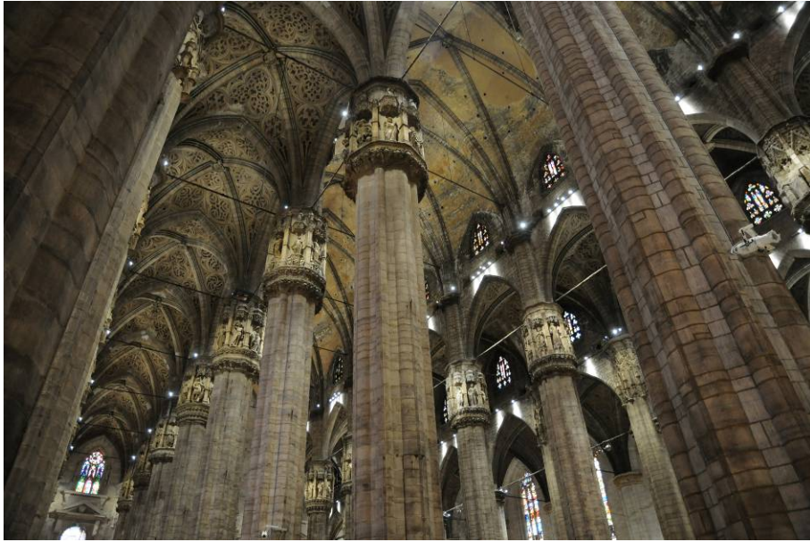
Fig. 4 View of the piers and of the tie-rods inside the Milan Cathedral
