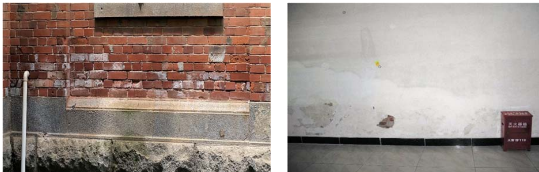
Figure 11, 12 (from Left to Right): Efflorescences and Salt Crusts phenomena are extensively present on the totality of the lower part of the façades; Raising Dump related Decay episodes are also present on many indoor walls
