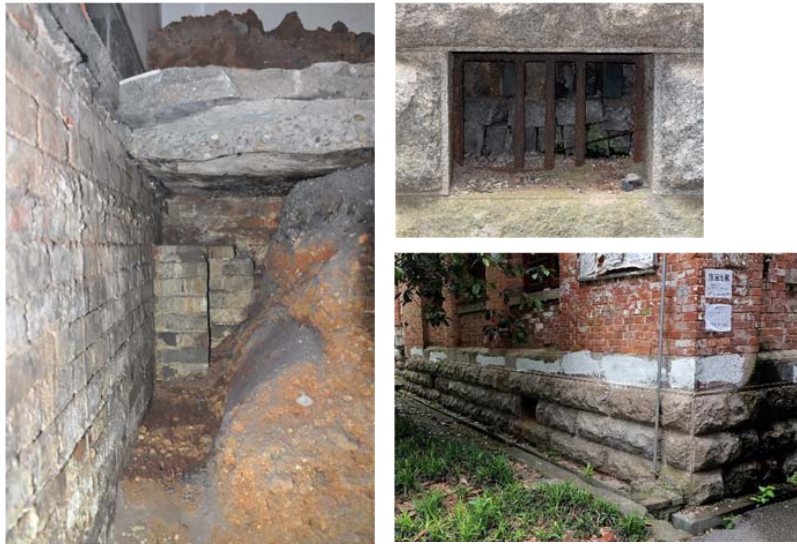
Figure 13, 14, 15: (from Left to Right, Top to Bottom): One of the diagnostic tests realized unveiling the land filling realized to build the ground level floor slab; A detail of one of the closed technical shaft windows; The technical shaft seen from the South-Eastern corner of the Building
