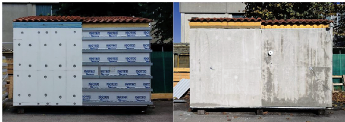
FIGURE 1. Test facility box installation phase of: (left) EPS insulation (West chamber) and micro-ventilated façade with Isotec ® wall (East chamber); (right) finishing layers equal for both chambers.
