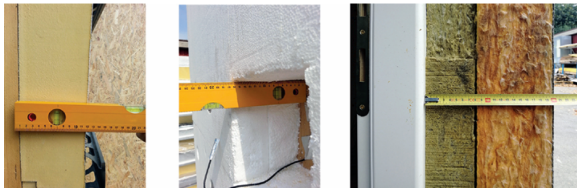
FIGURE 3. Zoom on thickens insulation during installation on the chambers. Left: Polyurethane foam Isotec® wall; Center: EPS panel; Right: double panel in high density rock wool.
