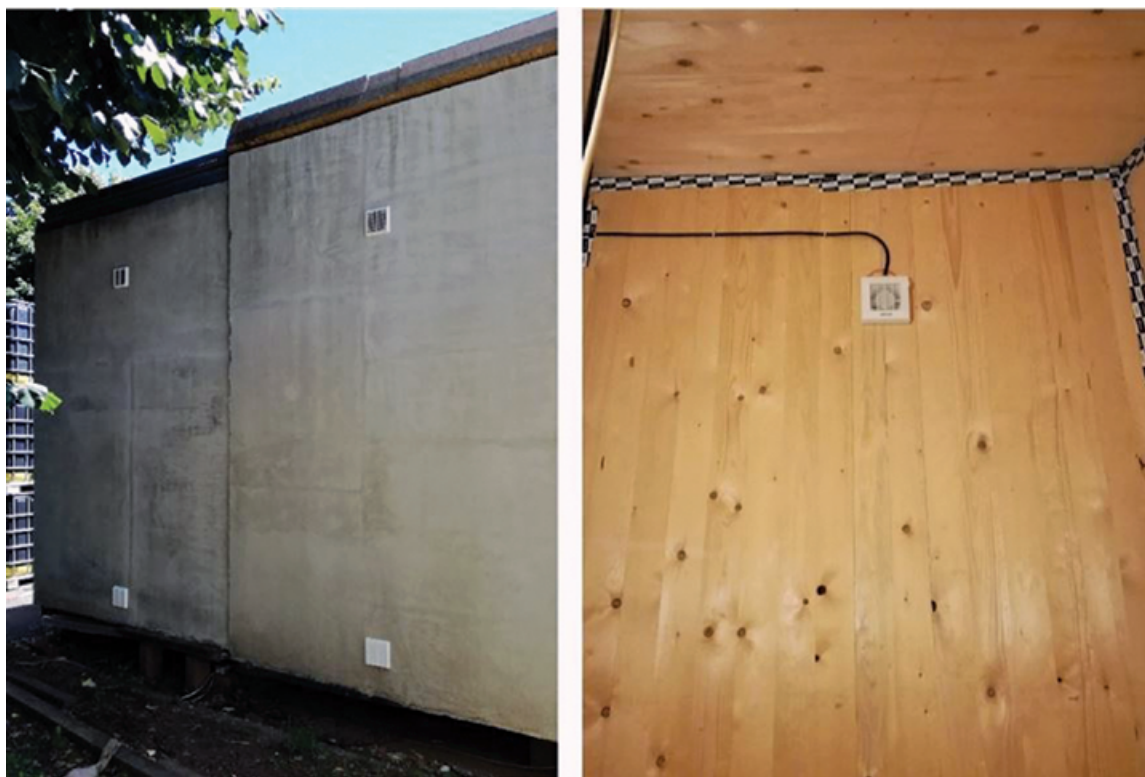
FIGURE 10. North façade of the text box. The white elements are the ventilation extract fans and the ventilation grilles.
