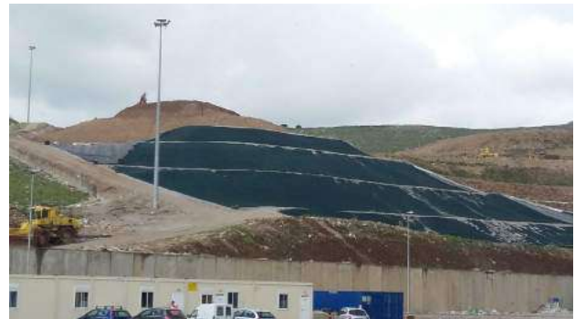
Figure 3. HDPE used as cap for the sector #1 and sector #2 of the landfill #6 (from RAP S.p.A. website).
