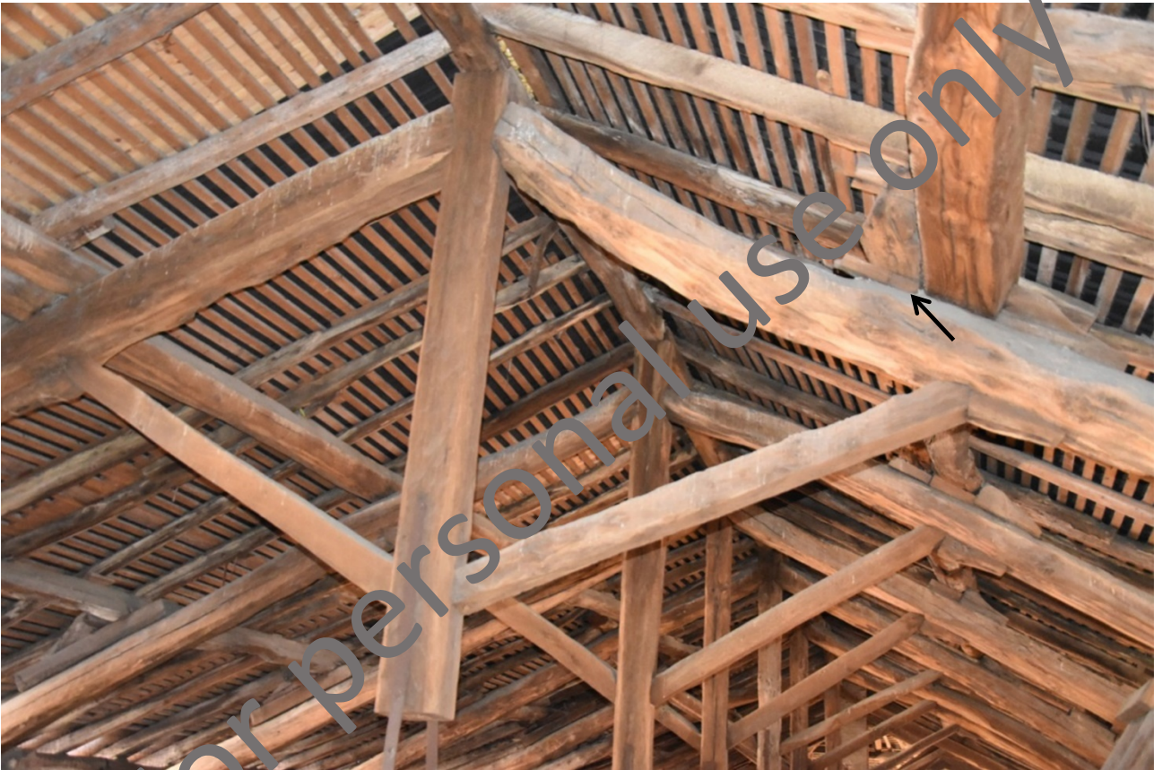
Figure 6. Wedges adopted to recover contact at the rafter (right rafter and purlin).
