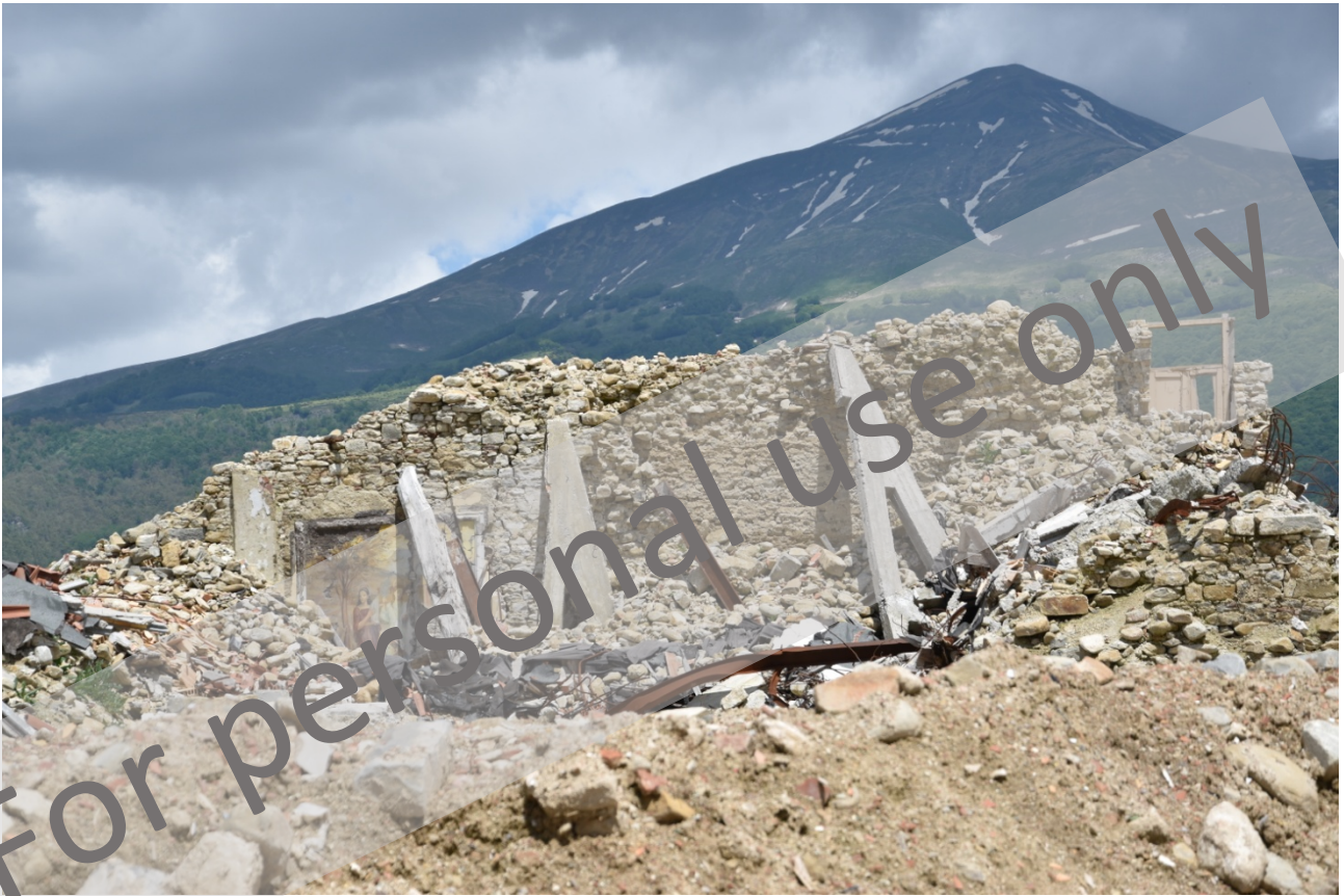
Figure 8 - Collapse due to massive intervention substituting timber trusses with concrete products at Amatrice, Central Italy earthquake, 2016.
