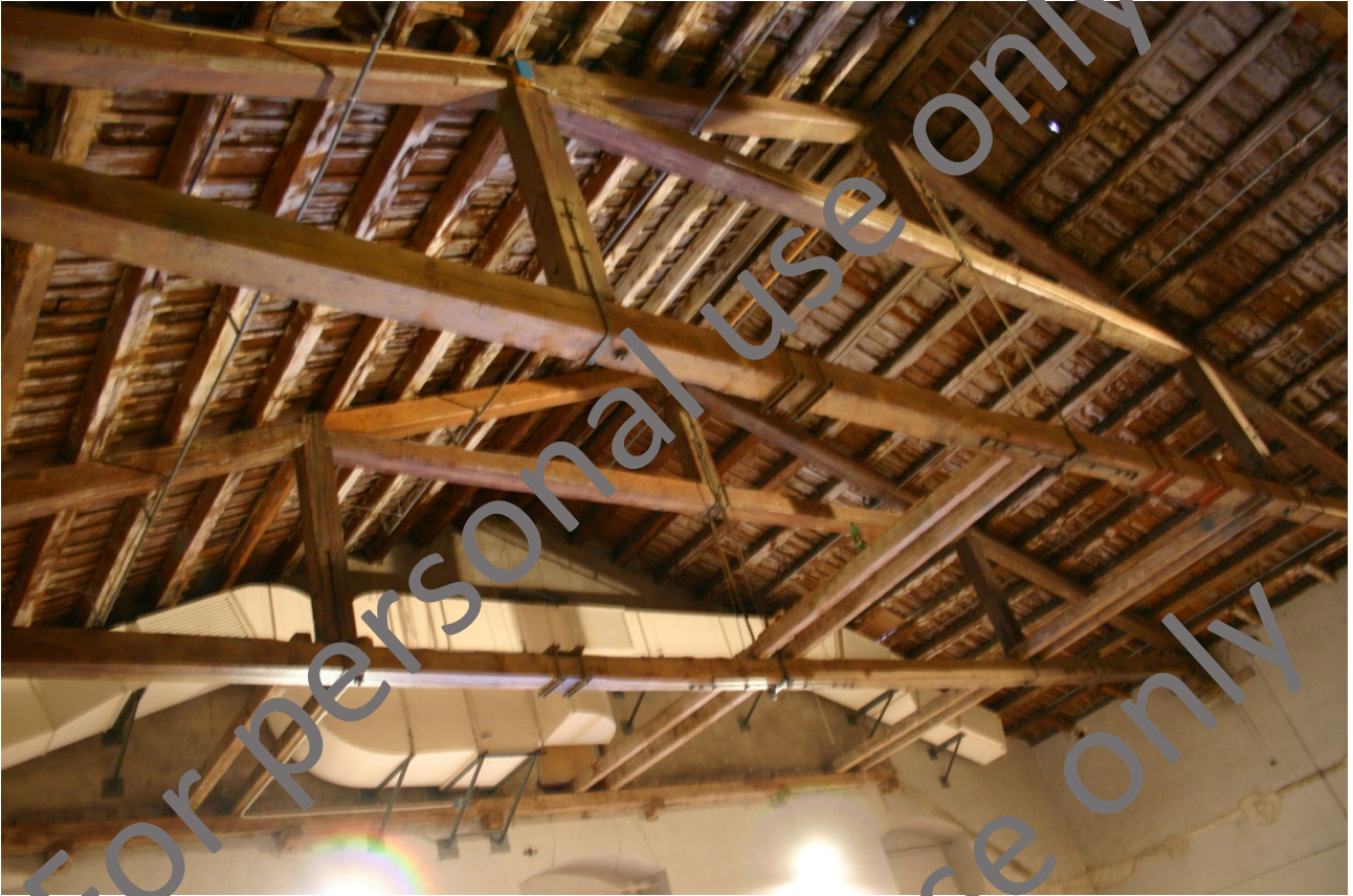
Figure 2. Queen-post truss with potentially unstable layout.
