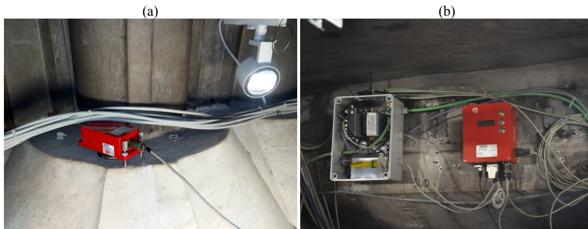
Fig. 6. (a) Seismometer and (b) digitizer installed in the Cathedral.
