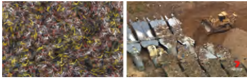
[Figure 5] Example of waste disposal in land fills: (Source: The Atlantic 2018 http://bit.ly/2JLZ4Ph )
