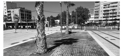
Fig. 3 - Pavement cooling through water circulation in Nice (source: https://www.2ei.veolia.com/en/our-main-projects ).
