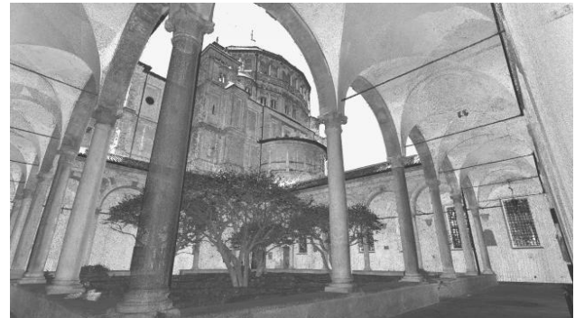
Figure 3. Point cloud of the Cloister of the Frogs, acquired by the Leica HDS 7000 laser scanner.
