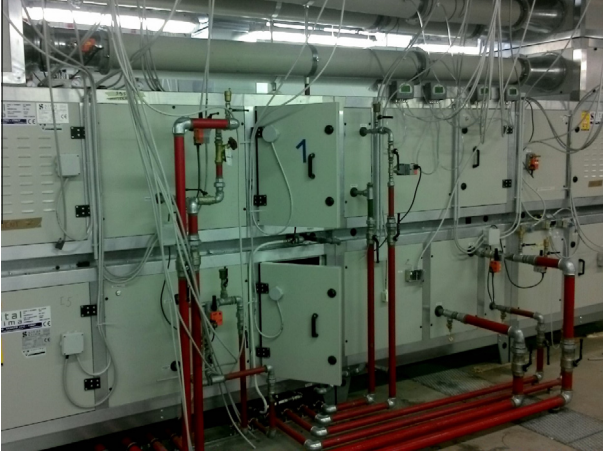
Fig. 3. Air handling units of the test rig.
