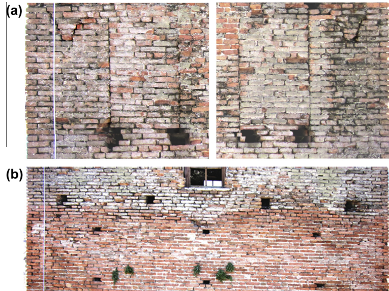
Fig. 3. (a) Probable merlons embedded in the masonry texture; (b) change of the surface workmanship at about 8.0 m from the top.
