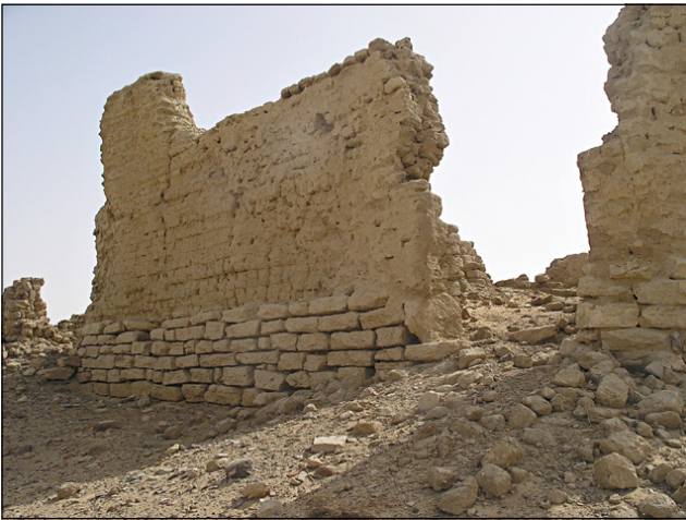
Fig. 9.3b – The western side of the central building resting on a stone basement (Photo by the Kharga Inspectorate staff).
