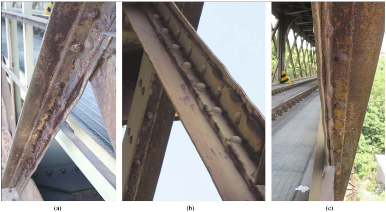
Fig. 4 Examples of the damage inflicted by the corrosion to the bridge members
