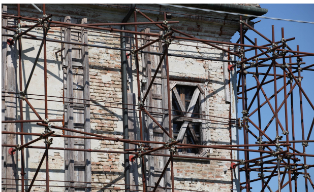
Figure 3: Building detail taken with the Canon telephoto lens. This lens allowed obtaining less distorted images of the upper part of the building.
