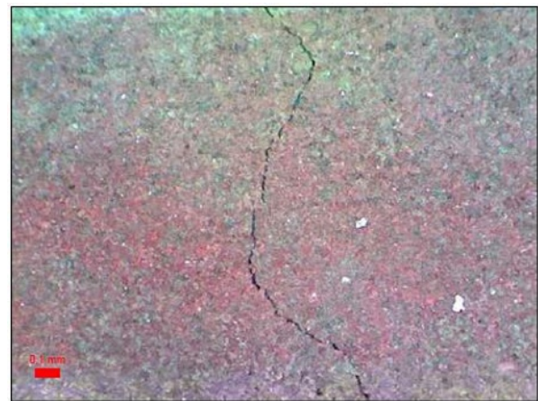
Fig. 6 – Crack of 0.01 mm in an UHPFRC at 200x magnification
