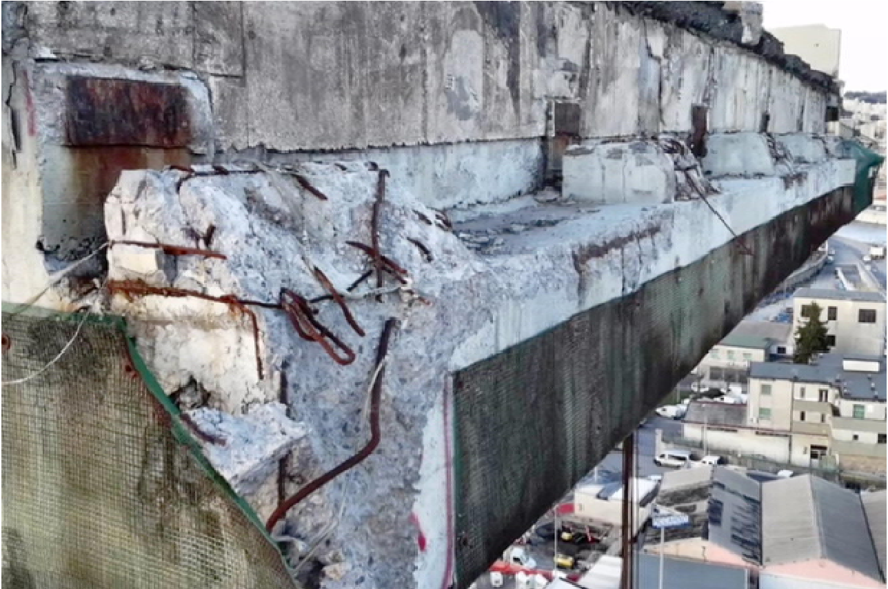
Figure 2 Detachment of the concrete cover, carbonation and oxidation of the reinforcements
