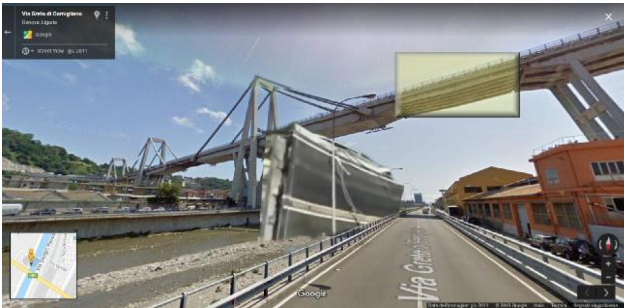
Figure 14 The position of the deck beyond the street lamp Cornigliano bank river road [Nota 10 ]
