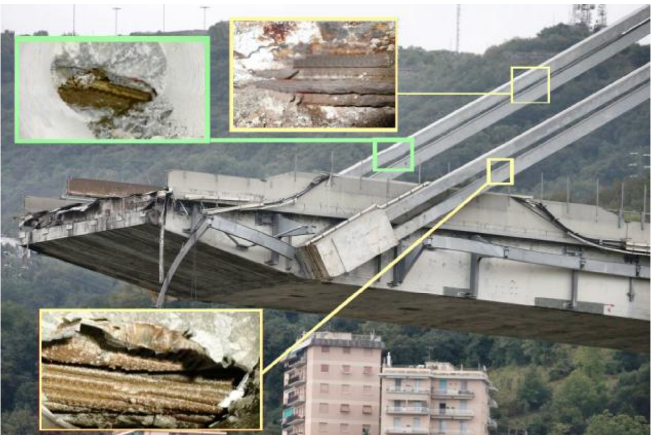
Figure 4 [Source Spea Engineering - January 2016] Diagnostic investigations on the stays of stack 9 and stack 10. The carrot carried out shows oxidation in the strands, corrosion and breakage of prestressing cables. The protective sheath is oxidized inside. Corrosion of the internal tie rods in the stay of the pile 10. The carrot investigates only secondary armor [Note 3].
