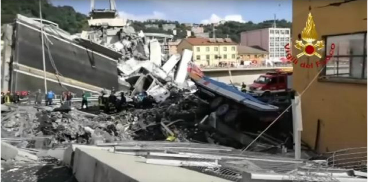
Figure 13 Collapsed roofs of some warehouses under the Morandi Viaduct
