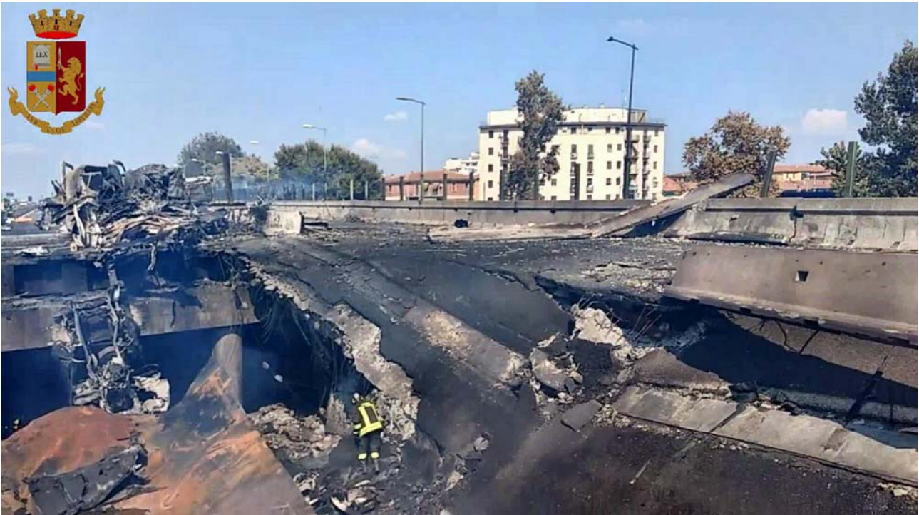
Figure 11 The road viaduct after the explosion
