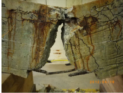
(a) Failure of corroded beam B2C13-1
