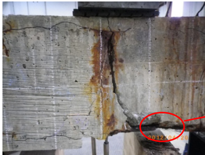
(b) Failure of corroded beam B2C13-2
