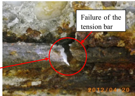
(c) Failure of tension bar of B2C13-2
