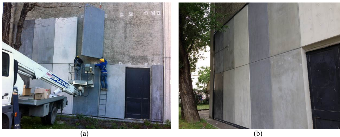
Figure 1– Test façade at Politecnico di Milano: erection of the façade (a) and the completed façade (b).
