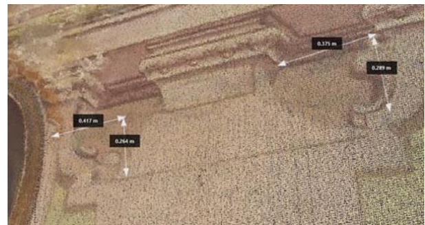
Figure 12. RGB three-dimensional view of the dense cloud: detail of the chromatic differences of the plaster in the points where the chains have been removed.
