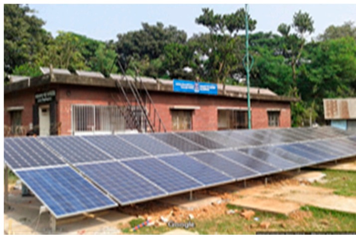
Figure 1. Solar PV panels in the University of Dhaka.
