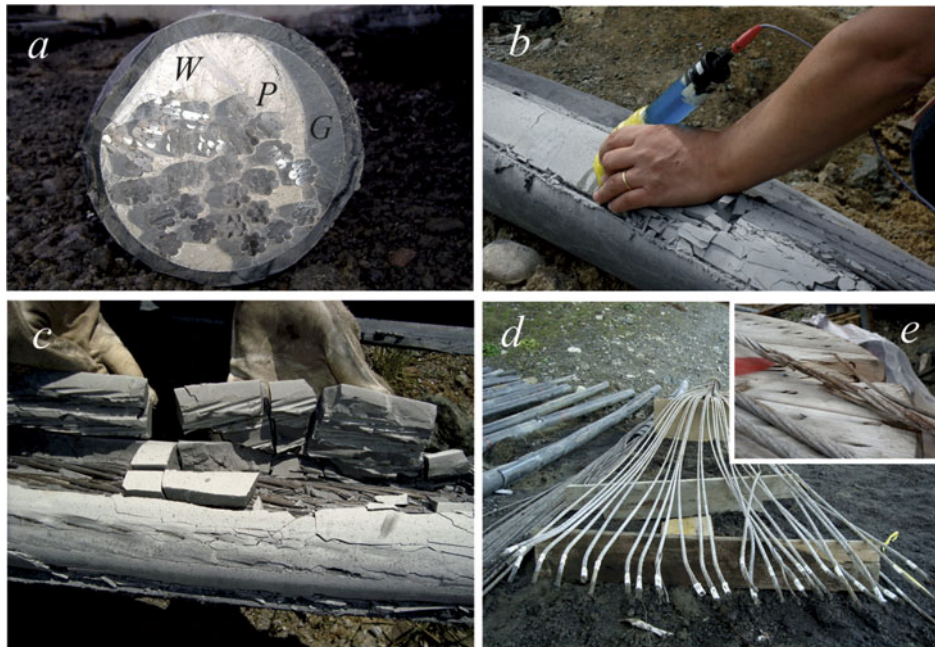
Figure 8. Inspection of a tendon removed from the bridge: (a) types of grout observed on a cutting section, (b) measurement of the corrosion potential of steel strands, (c) inspection of the grout, (d) inspection of the steel strands and (e) detail of wires of a strand broken due to corrosion.
