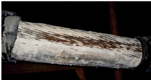
Figure 5. Example of an aperture in the duct of a tendon showing the whitish segregated grout embedding corroding strands.
