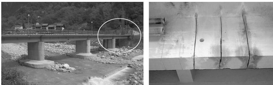
Fig. 3. General view of the Dogna Bridge (left, tested span circled) and detail of damages D1-D6 (right).
