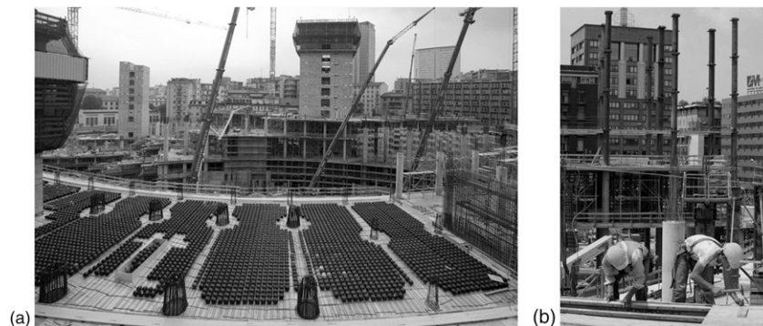
Fig. 3. Structural details (photos by Piero Mollica, Infrastrutture Lombarde S.p.A Archive; reproduced with permission): (a) bubble decks in Core 1; (b) steel encasing for columns of Core 1
