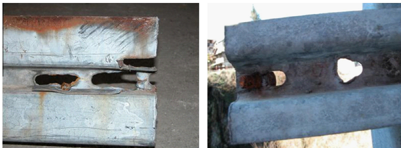
Fig. 7. Detail of the collapse due to plate bearing stress in the D joint. On the left the part of joint belonging to the CD segment, on the right the part of joint that remained in situ.
