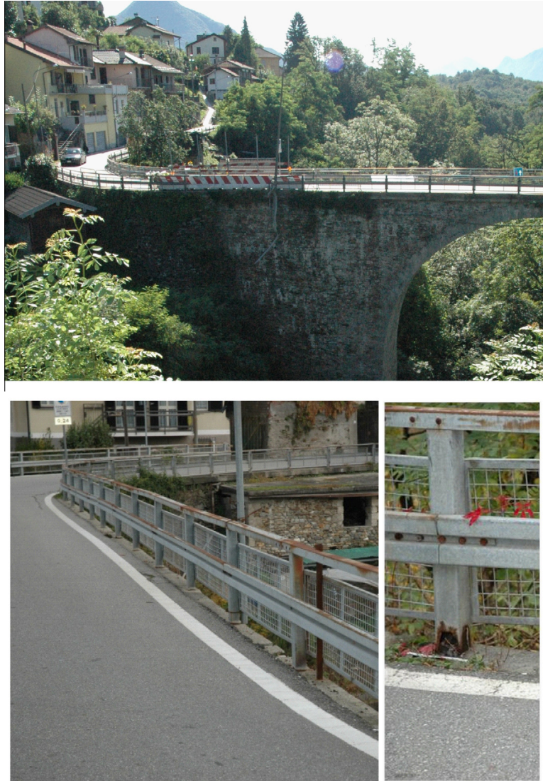
Fig. 1. Photos of the accident site (above), of the support guardrail posts (bottom left) and image in detail of a severe deterioration at the base of a post (right).
