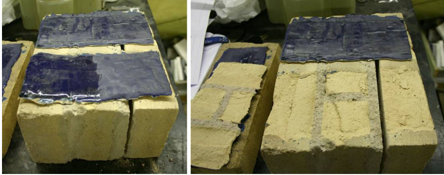
Fig. 5 Damage observed in the specimens after 40 thermal cycles; detail of the trimmed section
