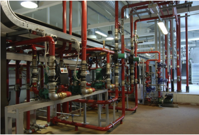
Fig. 3. Hydraulic plants above the test room.
