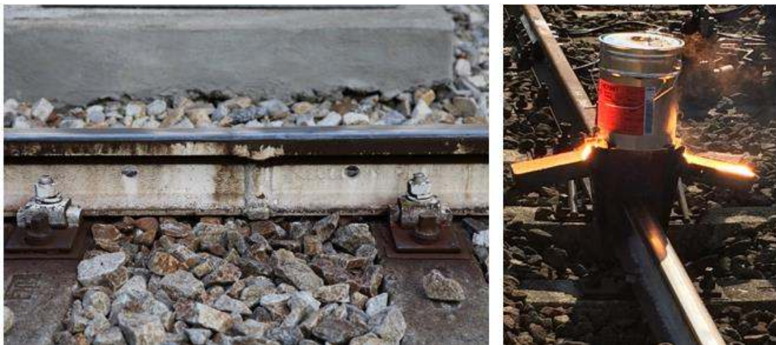
Figure 1. The “long welded rail”.
