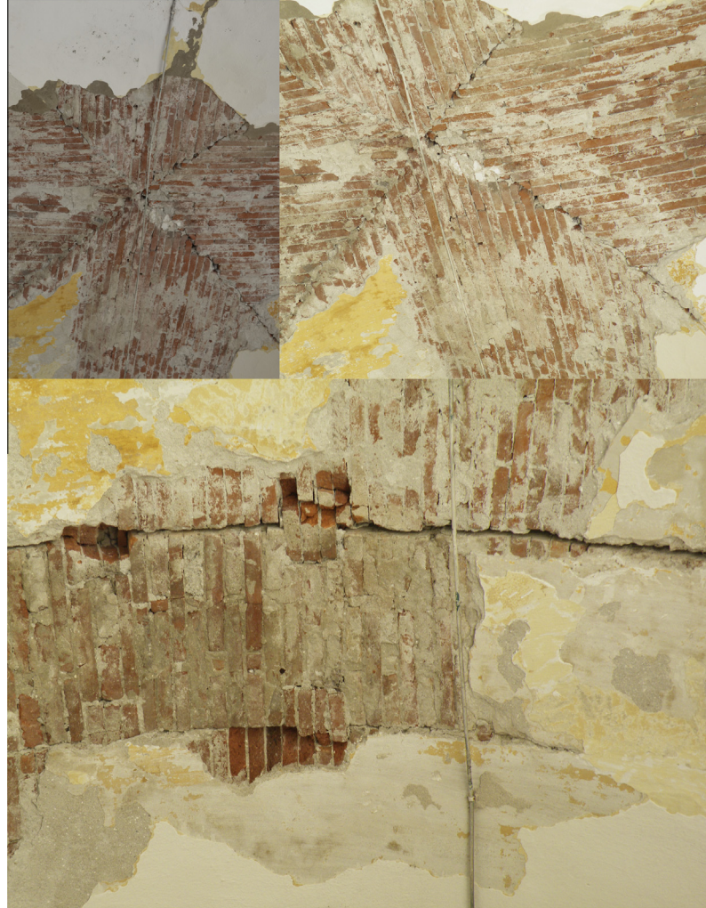
Fig. 3. Existing state of damage. Diagonal cracks (top) and full detachment of the lateral ribbed arch (bottom).
