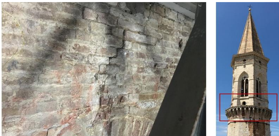
Figure 3: Cracks in the lower part of the belfry.
