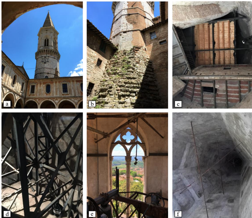
Figure 2: San Pietro bell tower: a) North-West side of the tower; b) Basement; c) Interior of the tower; d) Metal structure supporting the bells; e) One of the mullioned window; f) Interior of the cusp.
