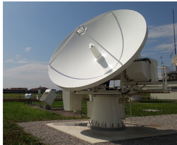
Fig. 4. Alphasat ground station in Spino d'Adda pointing at the Alphasat satellite.
