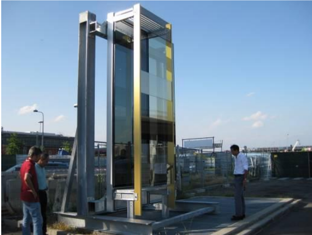
Figure 9. Production of the “double skin façade” mock up (5+1AA and Jean-Baptiste Pietri Architectes, Office Building, Rho, Milan; construction drawing).
