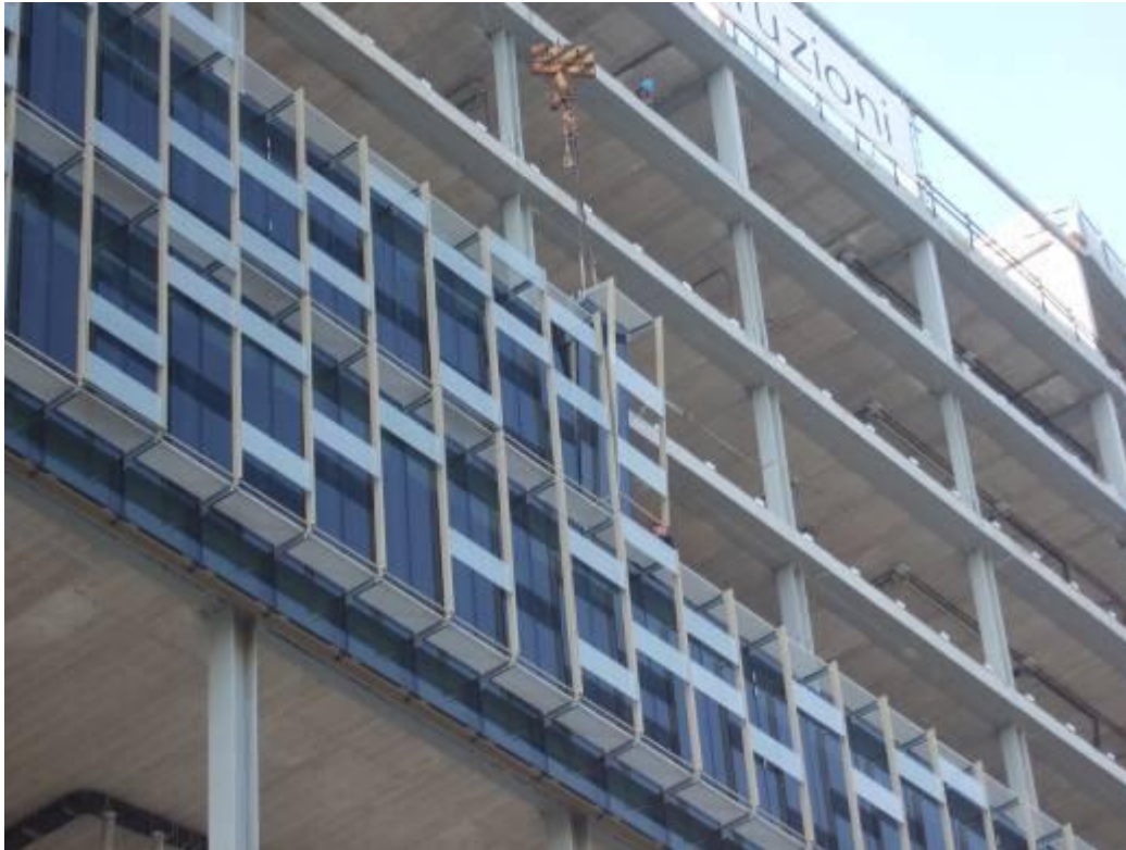
Figure 10. Construction phases of the “double skin façade” components (5+1AA and Jean-Baptiste Pietri Architectes, Office Building, Rho, Milan; construction drawing).
