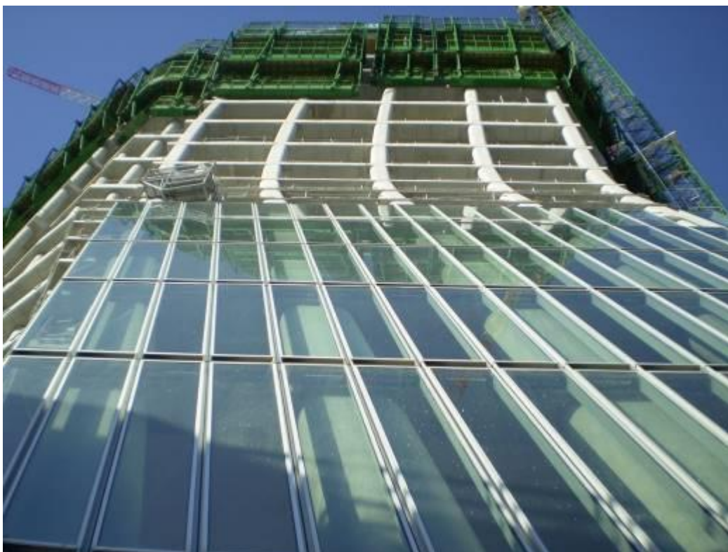
Figure 7. Construction phases of the “unit system” building envelope (Zaha Hadid Architects, CMA-CGM Tower, Marseilles; construction drawing).
