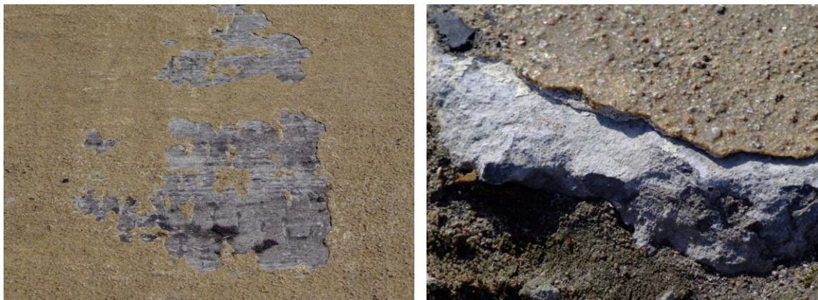
Figure 2. Improper choosing of repair material (too strong and too stiff) in retrofitting of an airfield pavement. Left: View of a spalling PC cover from an old runway made of weak concrete. Right: Detail of failure in the repaired concrete substrate, caused by thermal incompatibility. Credits: B. Zajac.
