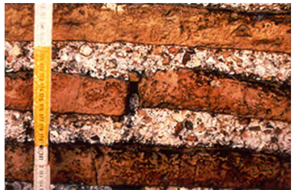
Fig. 13 View of thick mortar joints of St. Vitale basilica in Ravenna (Italy)
