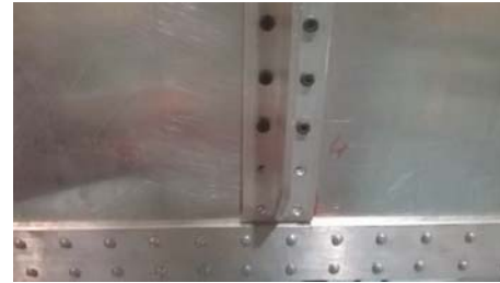
FIGURE 7: Detail of D5 damage.
