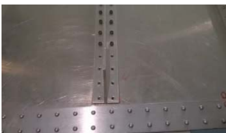
FIGURE 5: Detail of D2 damage.
