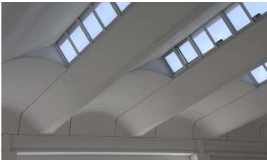
FIGURE 1. Roof of precast dry-assembled industrial building made with spaced wing-shaped elements with zenith light openings
