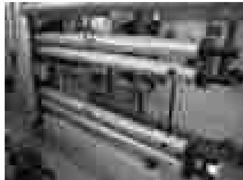
Original heat exchangers in the boiler room (before renovation). [2]
