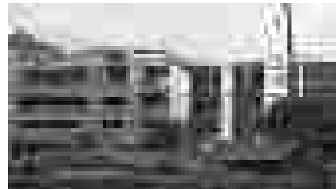
Left building part already renovated – right building part in the middle of the renovation
