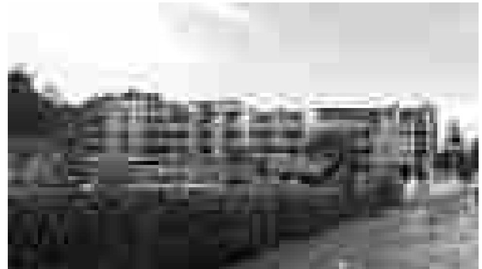
A few days later – building envelope of the right building part almost finished
