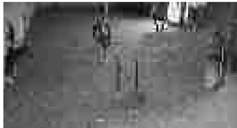
Photovoltaic system - TNT under flooring above systems
