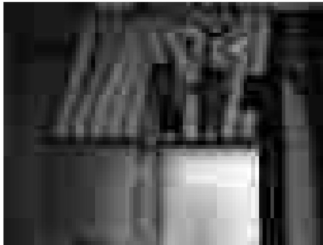
Distribution section of mechanical ventilation system.
