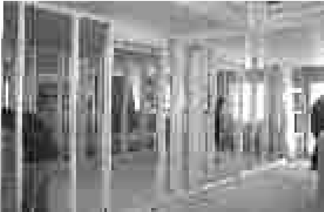
New internal walls and inserted deck at the first floor of block B.
