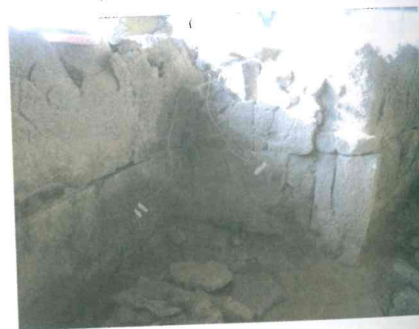
Figure 6 Interior of the main room, positioning of the surface temperature probes S2 1-4
