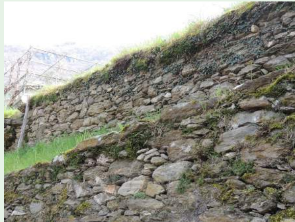
Fig. 29 - In the foreground, the junction of a previous wall to a new part. (photo: Andrea L'Erario)
