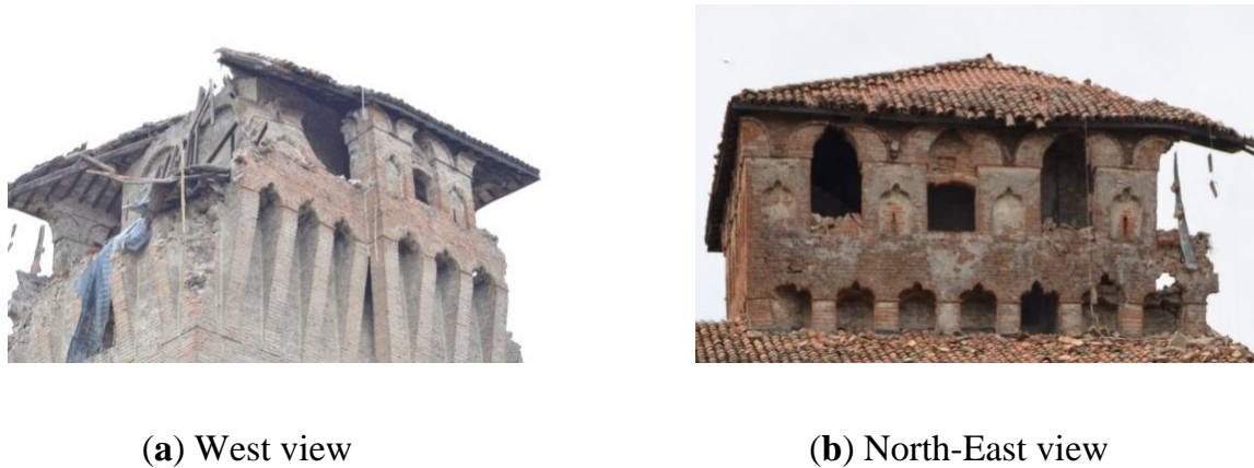
Fig. (7). Damages on the West tower crown, where partial collapses were observed.
