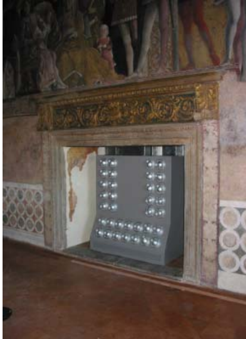
Fig. 5 – Picture of the air diffusers placed inside the fireplace of Camera Picta without the visual shielding grid.
