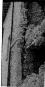
Figure 1. Separation of masonry leaves and collapse under out of plane actions
