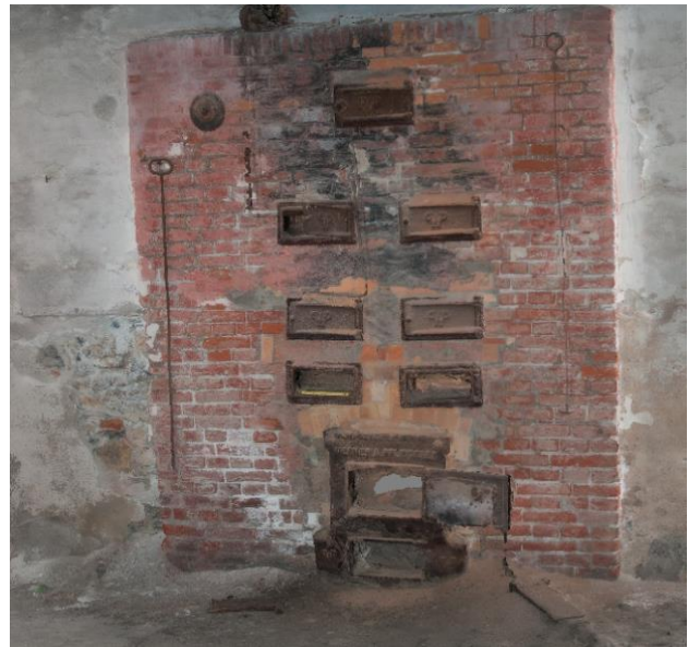
Figure 6. Tiled model view of case C, a wall of the ovens in the kitchen of the Albergo dei Poveri .
