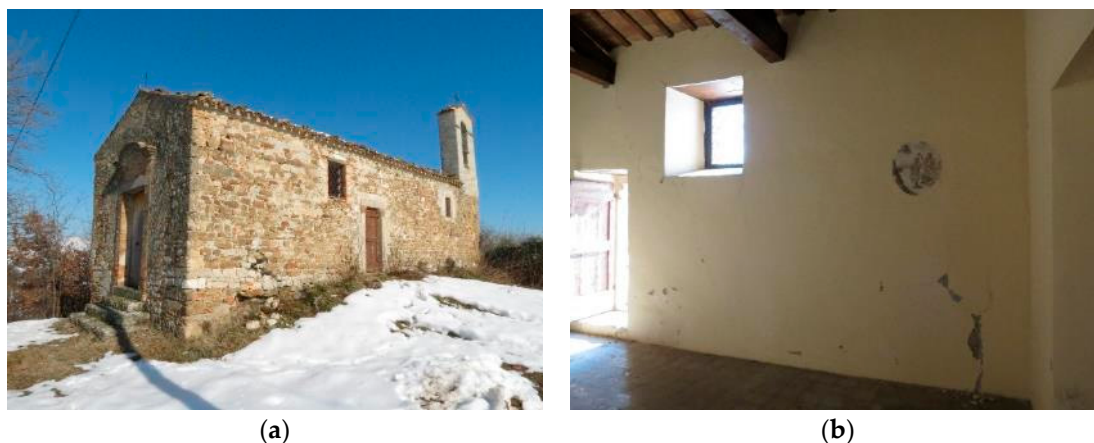
Figure 7. Example of damage due to soil settlement occurring after a seismic event: (a) visible outside a church; and (b) inside a church.
